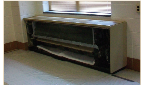
PHOTO 2 School fan coil unit.
