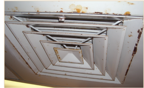
PHOTO 4 Rusting diffuser from over-cooling.
